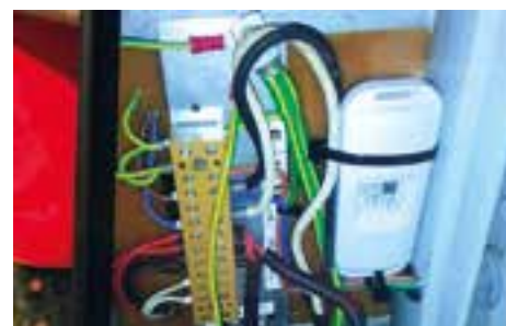
The Disruptive Technologies wireless sensor inside an electrical box on a rig
